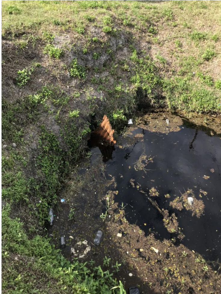
Collapsed side drain at Savannah Road outfall ditch
